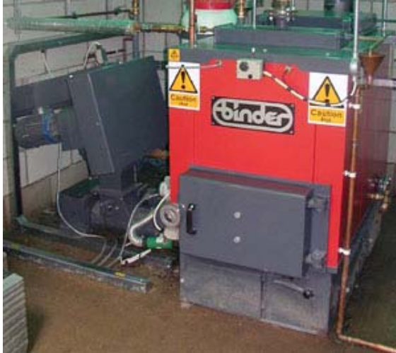
Figure 6. Binder (50kW) wood chip boiler meets 50% of large educational centre's hot water demand
